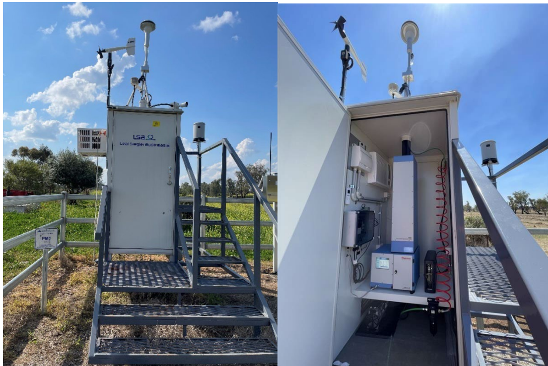
Figure 1: TEOM installed at Lanreef
